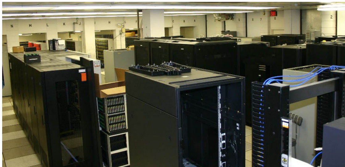
One of CNS's Machine-Rooms
